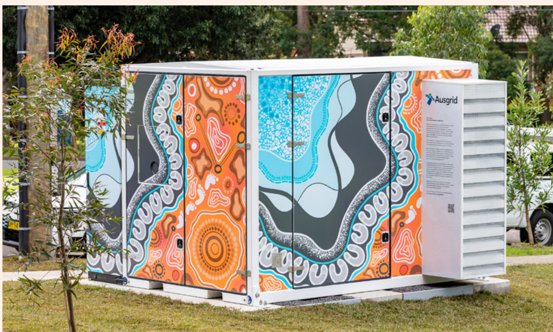
A community battery in Bexley North, New South Wales. Photo courtesy of Ausgrid.
